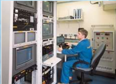
Typical interior of a Seaeeye Control Cabin
